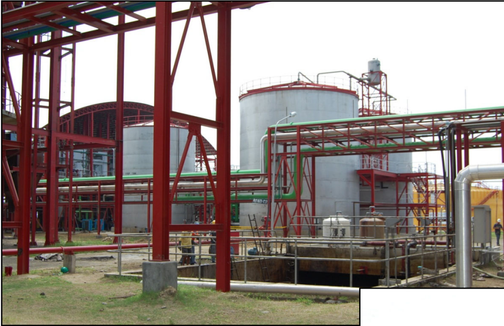
➤ Fuel Ethanol Distillery Plant (SCBI)
